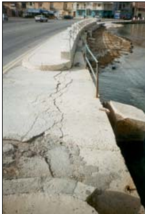
Fig. 7: Damaged road alignment at Xemxija showing remaining sandy pocket.
