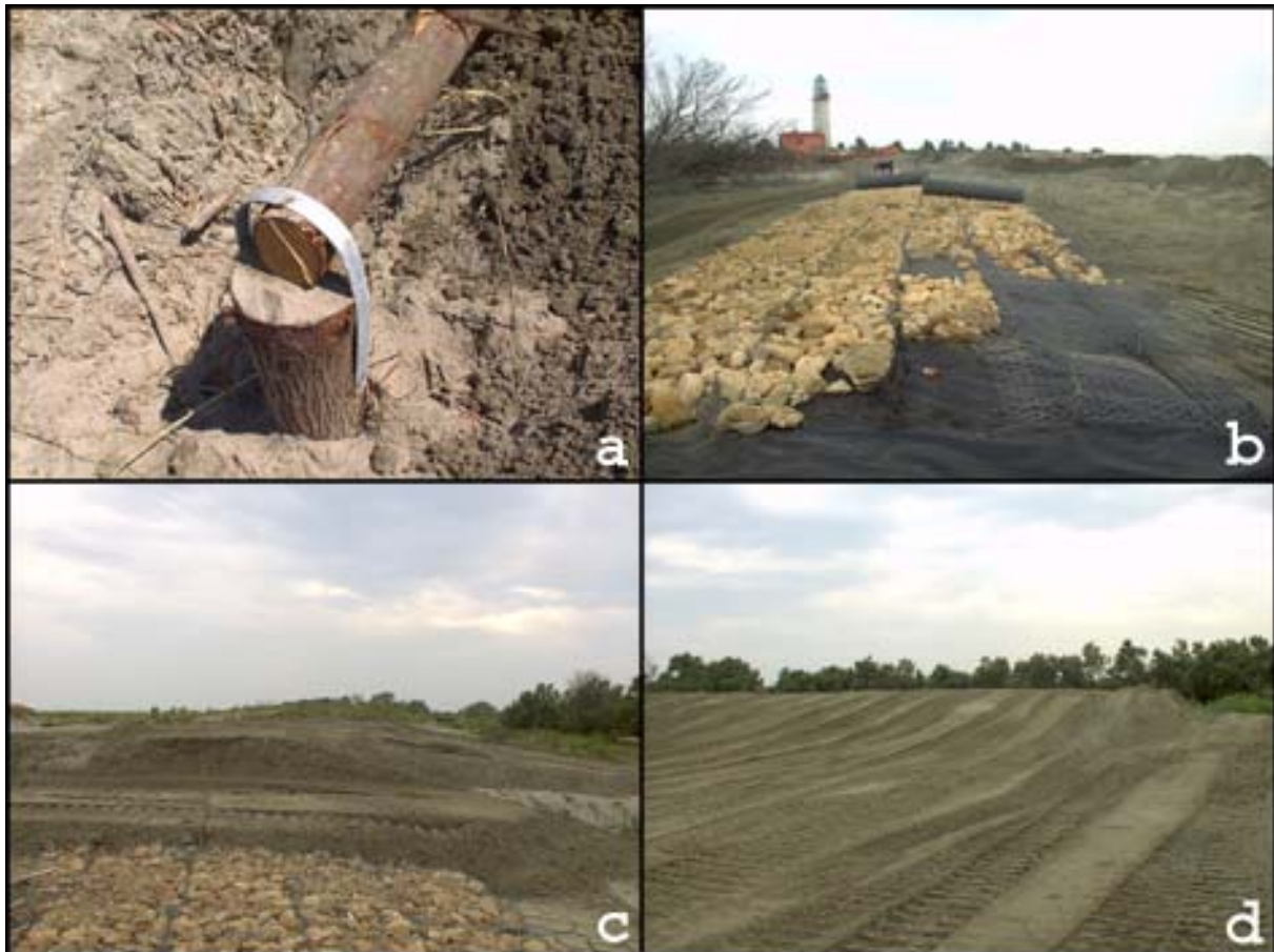
Fig. 9: The reinforced coastal dunes construction: a) the wood poles structure on what have been placed the gravel mattresses; b) the gravel mattresses under the sands shaped as dunes; c) the coastal dune building; d) the final armoured dunes shaping.
