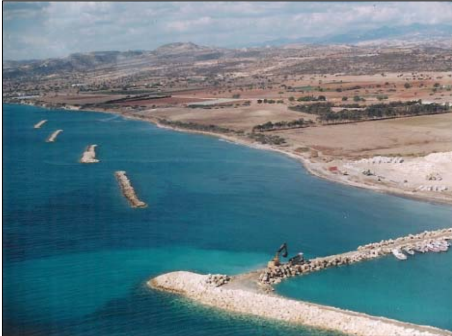
Fig. 9: Offshore breakwaters in Alaminos – view west. An harbour is being illegally constructed at the right bottom of the photo.
