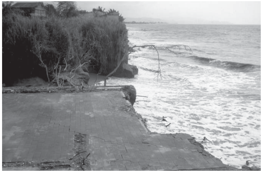
Fig. 5. The rapid retreat of the cliff bordering the Puerto Gaviota surface, due to undermining by waves during high tides, is affecting some cottages built too close to its edge at the time.
